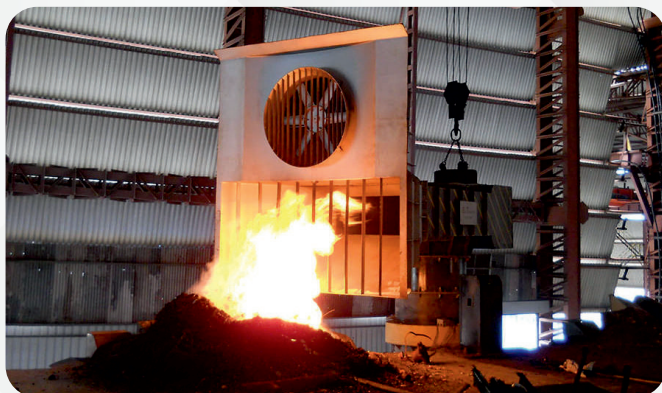
Air Polution Control System
